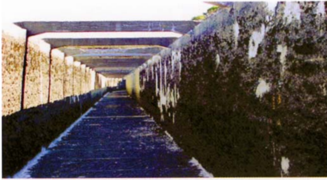
After 70 years of service, the Liawenee flume was in an unacceptable state (left). After refurbishment and cleaning
