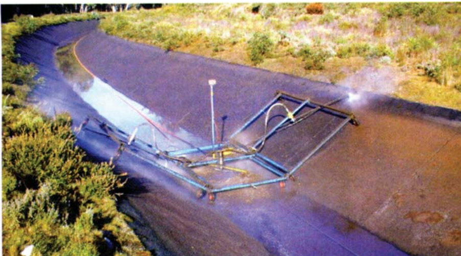
This canal scrubber, which consists of water jets on rotating arms mounted on a frame, was tested in early 2005 in the canal that supplies water to the 93.6-mw Tarraleah project. Each cleaning improved flow by 3 cumecs.
