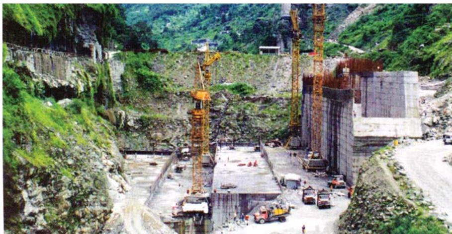
Construction of hydroelectric projects in India is accelerating. The government is calling for more than 50,000 mw of new hydro capacity to be added by the end of 2017.
