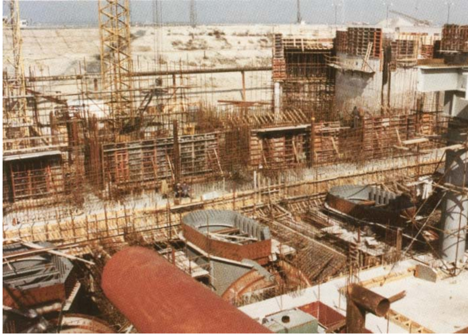
Worldwide, hydropower development is occurring at a rapid pace. More than 900 hydro projects currently under development will add 200,000 Mw of electrical generation capacity. (Photo courtesy Voith Siemens Hydro Power Generation)
